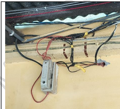
Photo: 100A Fuse at grid supply incomer
