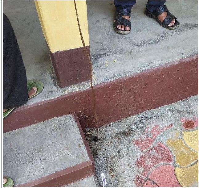
Photo: Earthing strip connected to the earth-pit buried underground.
